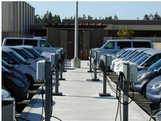
Figure 2. Vandenburg Air Force Base charging infrastructure.
