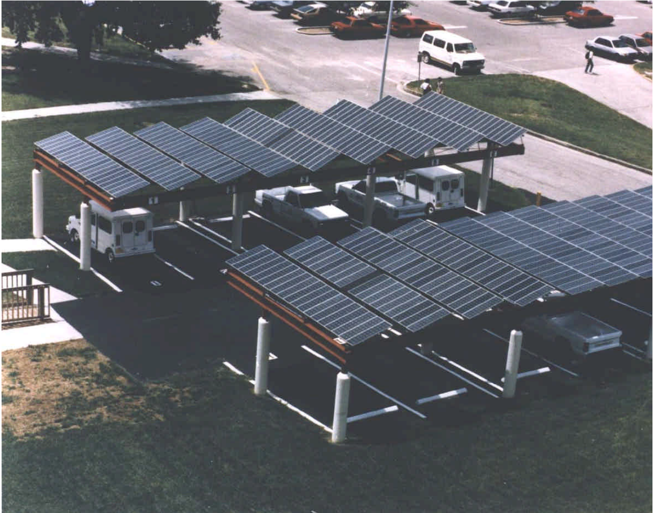
Figure USF-3. 20-kW solar energy charging station located on the campus of the University of South Florida up to 12 electric vehicles, using 377 Siemens 53-watt solar modules. When not charging vehicles, the electrical cells are fed into the local utility grid. (photo 95-943-1-1)
