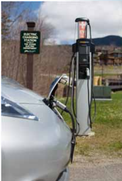
ChargePoint Level 2 EVSE in Stowe
