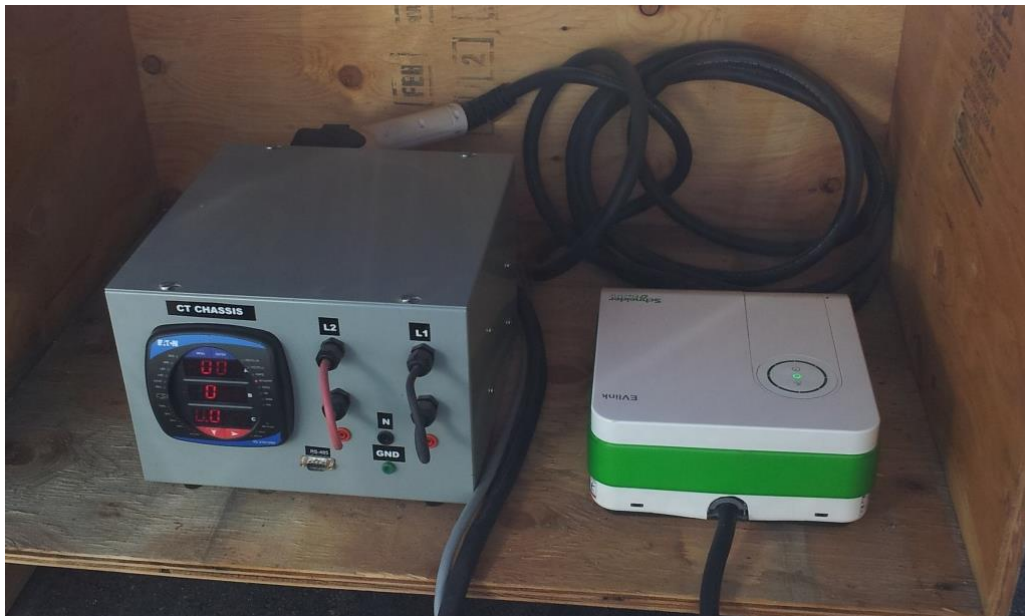
Figure 3. Schneider Electric AC Level 2 EVSE unit in series with Eaton IQ250 power and energy meter.
