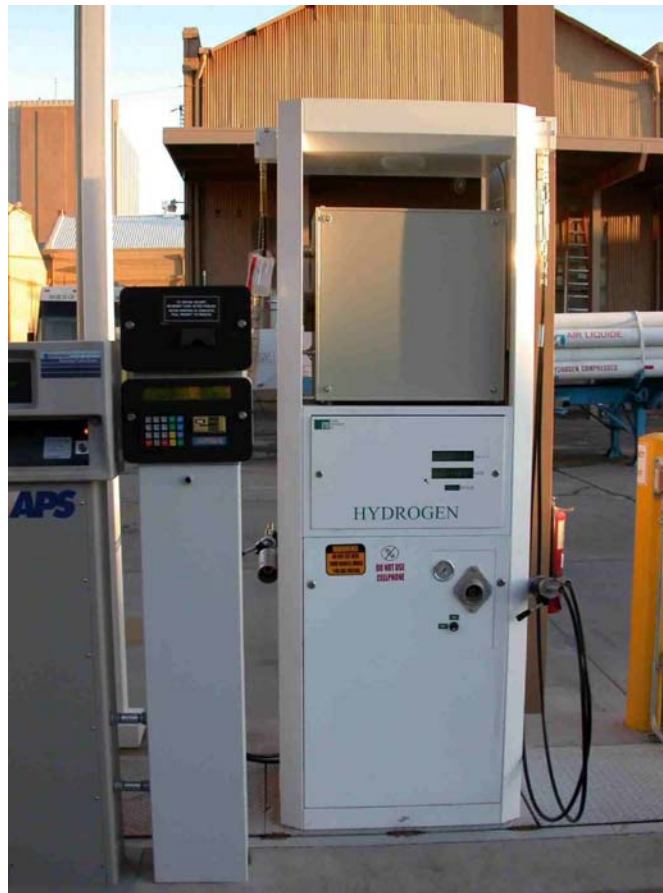
Figure 2; FTI Hydrogen Dispenser.
