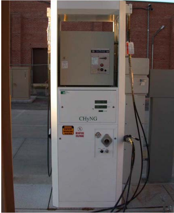
Figure 5. FTI blended fuel dispenser.
