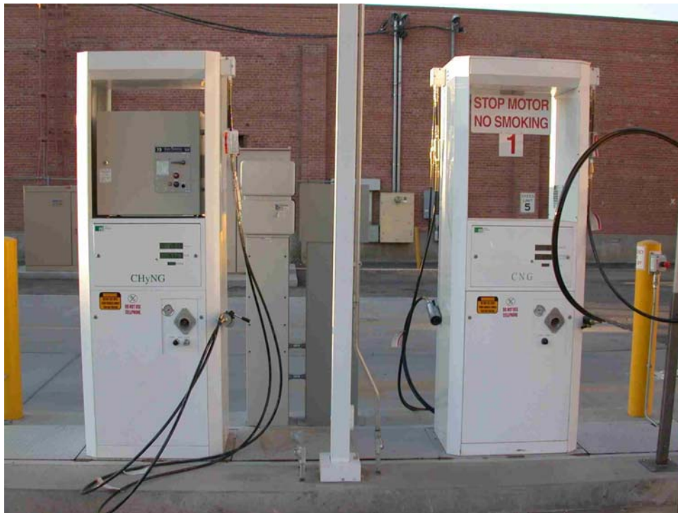
Figure 2. Fueling Technologies Inc. fuel dispensers (CNG and hydrogen/CNG blend fuels).
