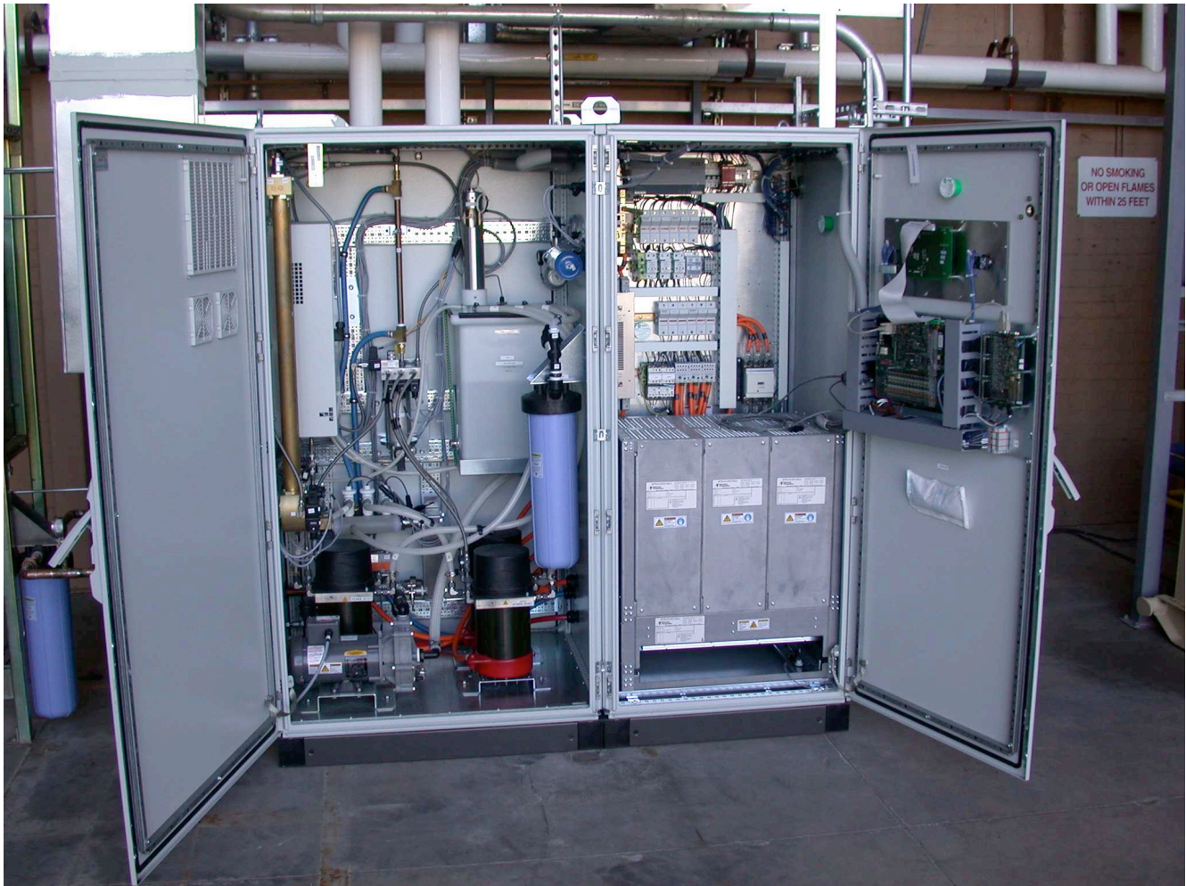
Figure 1: Hogen Electrolyzer Installed in the APS Alternative Fuel Pilot Plant
