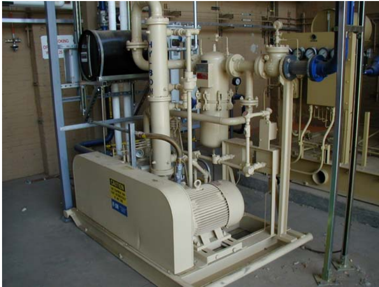
Figure 3.1. Hy-Bon - CNG boost compressor.
