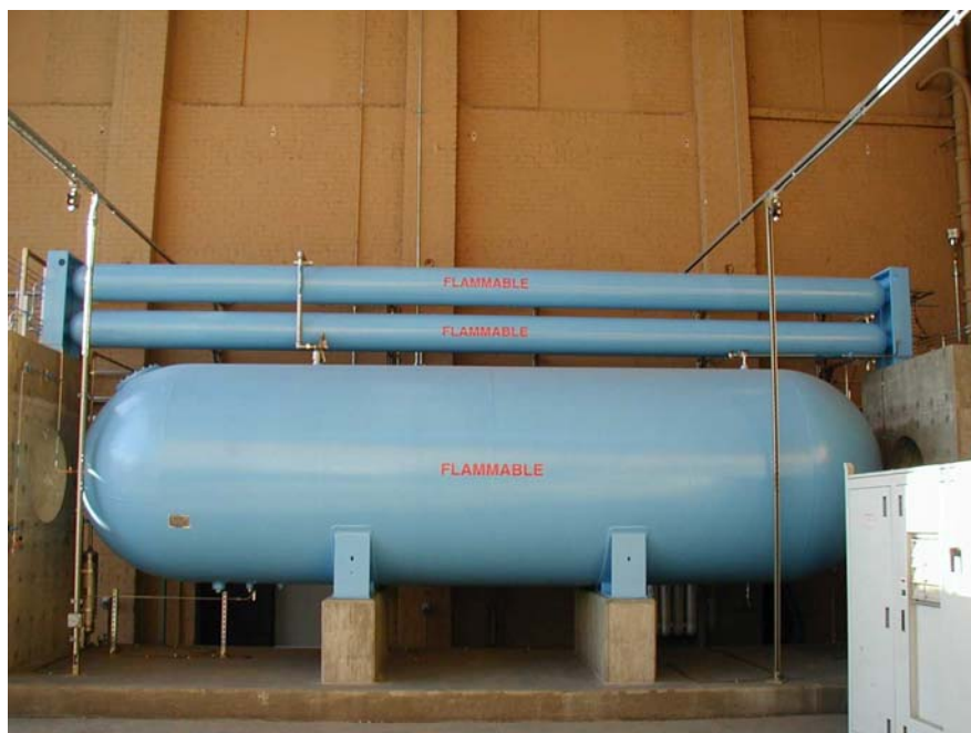
Figure 2.3. Hydrogen low-pressure storage vessel is the large tank on the bottom and the two high-pressure storage vessels are on top.
