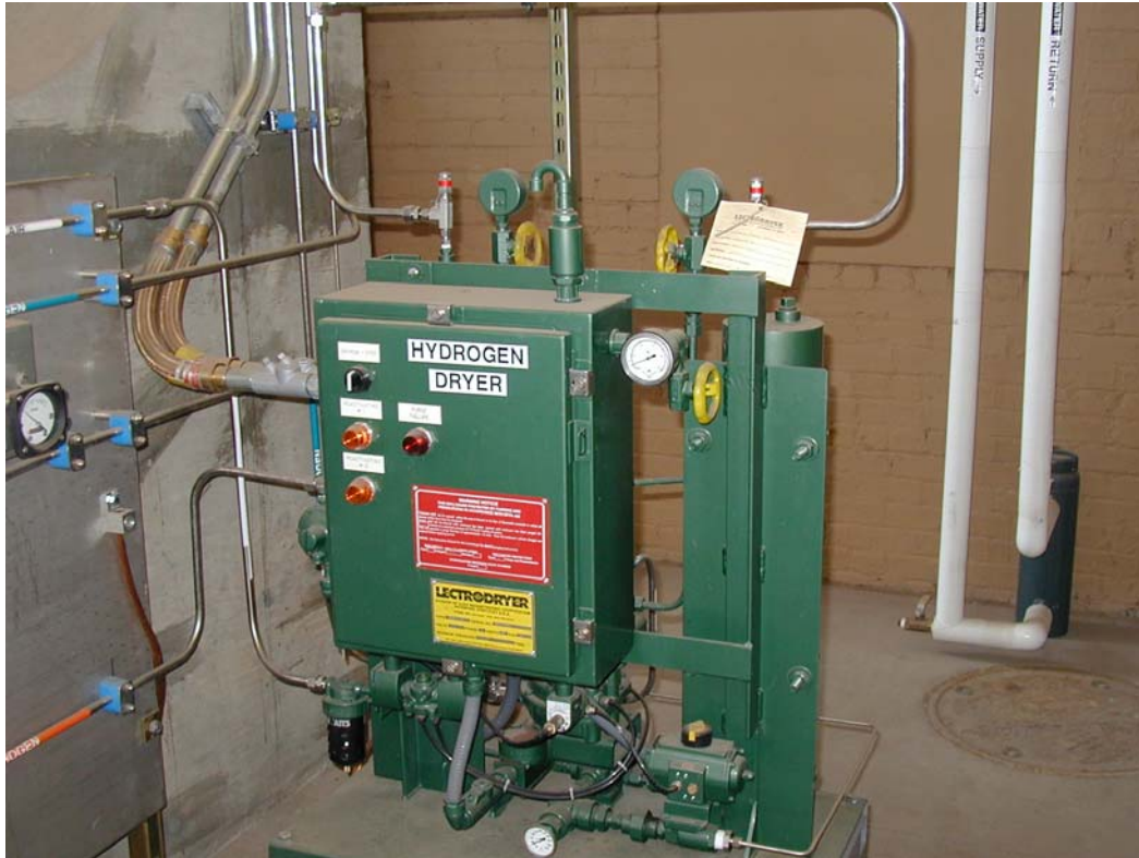
Figure 2.2. Lectrodryer hydrogen dryer.
