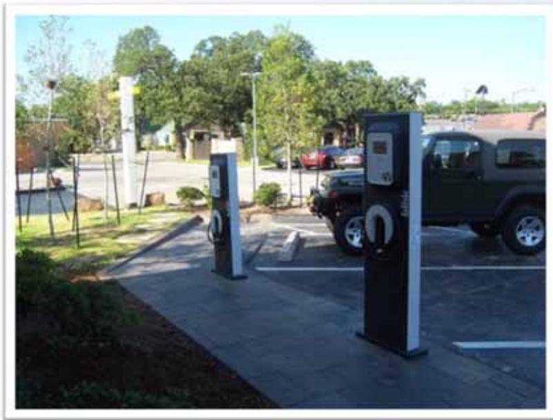
Pedestal EVSE installed on decorative paving ; removal and replacement required for underground conduit
