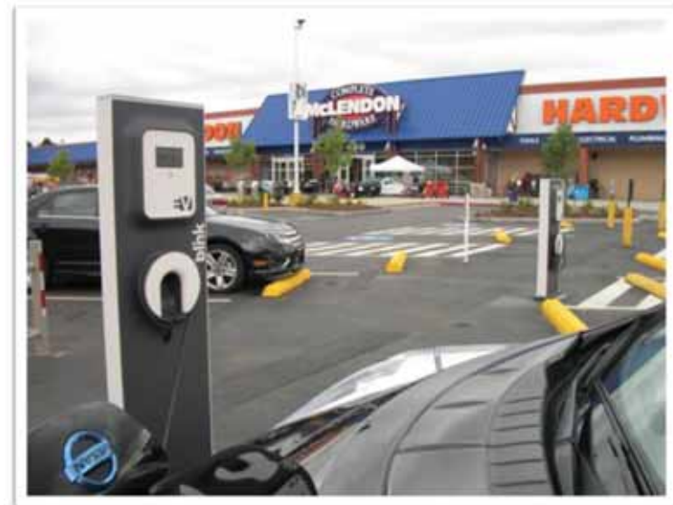
Pedestal EVSE installed on asphalt, with trenching and repaving for underground conduit
