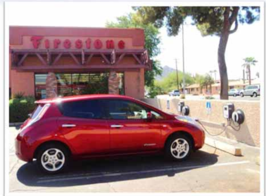
Wall-mounted EVSE installed on block divider wall with surface mounted conduit
