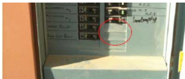
Figure 2. Circuit breaker panel and space for two circuit breakers to support Level 2 EVSE.
