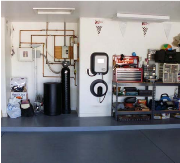
Figure 3. Clear floor and wall access to Blink EVSE.
