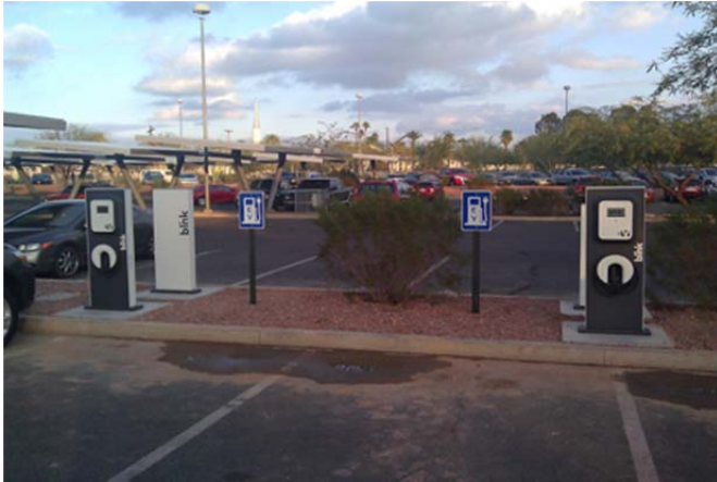
Figure 1. Combined visitor/employee charger installation.
