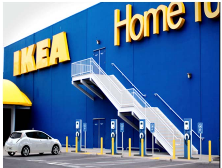
Figure 2. Retail EVSE installation.
