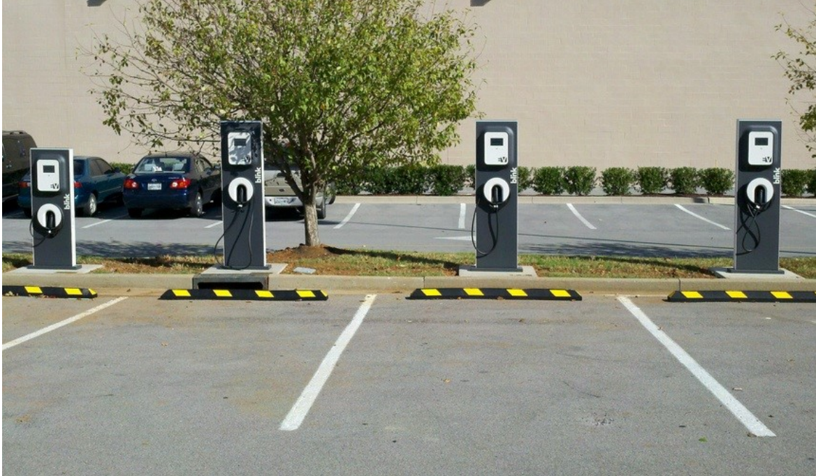
Figure 5. AC Level 2 EVSE mounted on precast concrete pedestals. These EVSE are intended to charge one PEV per parking spot. Note that the left most EVSE is of reduced height in order to comply with the American with Disabilities Act.
