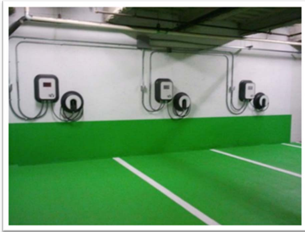
Figure 4. Wall-mounted AC Level 2 EVSE in a parking garage. These EVSE are fully functional and are a good example of a wall-mounted EVSE in a parking garage.
