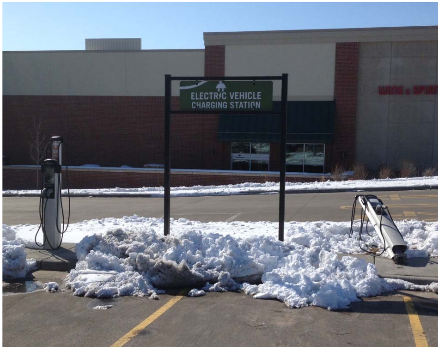
Figure 9. Fully functional AC Level 2 EVSE damaged by a snow plow.
