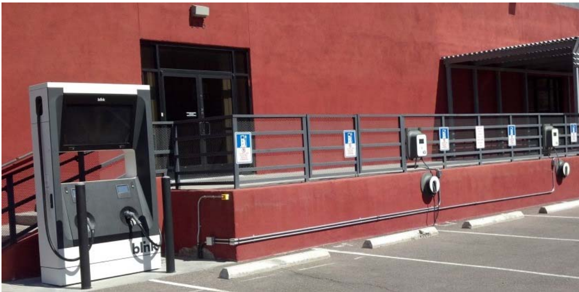
Figure 7. DCFC to the left and two AC Level 2 wall-mounted EVSE to the right.
