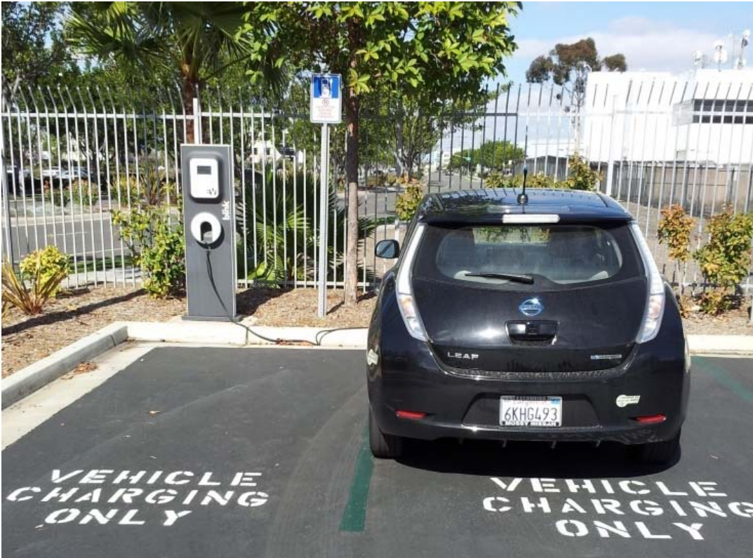
Figure 6. AC Level 2 EVSE mounted on a precast concrete pedestal. This EVSE is intended to charge vehicles in both parking slots.
