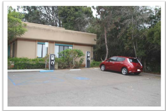
Figure 4. ADA-access compliant EVSE installation.
