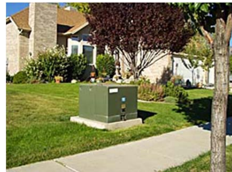
Figure 1. Pad-mounted residential distribution transformer. 2
