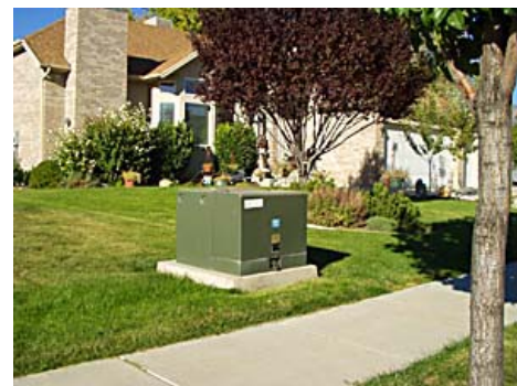
Figure 2. Pad-mounted Residential Distribution Transformer 1
