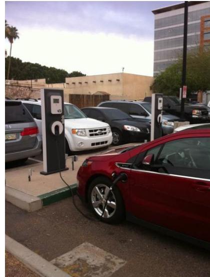
Level 2 EVSE Charging Station at Monti's la Casa Vieja, Tempe, AZ
